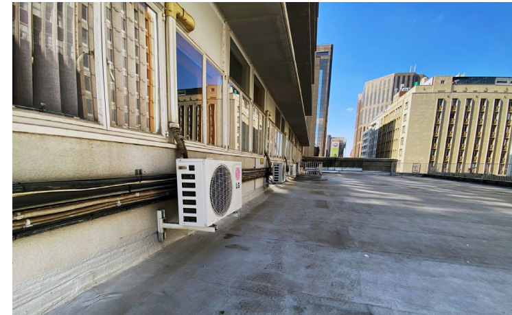
Images showing: 1)Air conditioning condensers. 2) Fire booster in the 1 st basement.
