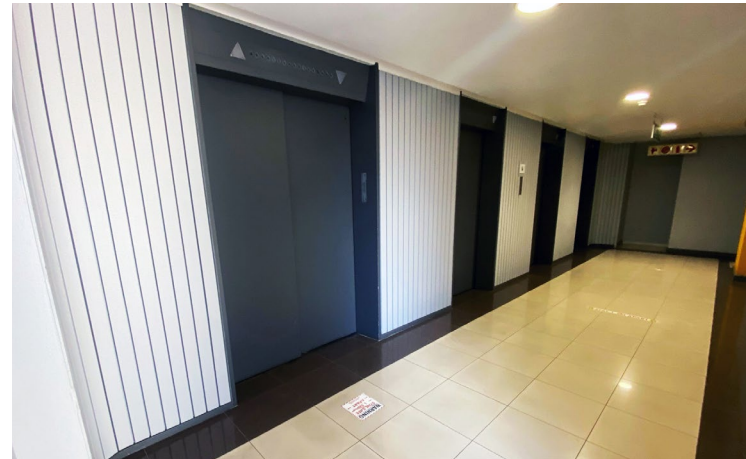
Images showing: 1) Goods Lift & Passenger lifts. 2)Passenger lift. 3) Interior of goods lift.
