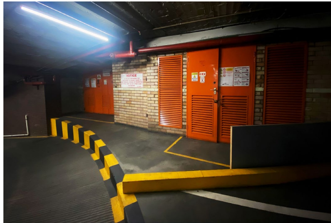
Images showing: 1)LT room in the 1 st basement. 2)Backup generator.
