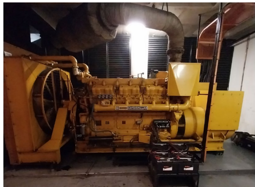
Images showing: 500Kva Generator
