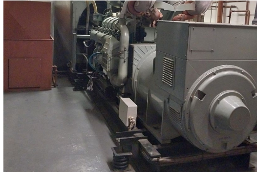
Images showing: 800Kva Generator
