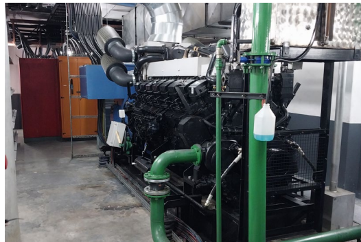
Images showing: 1900Kva Generator
